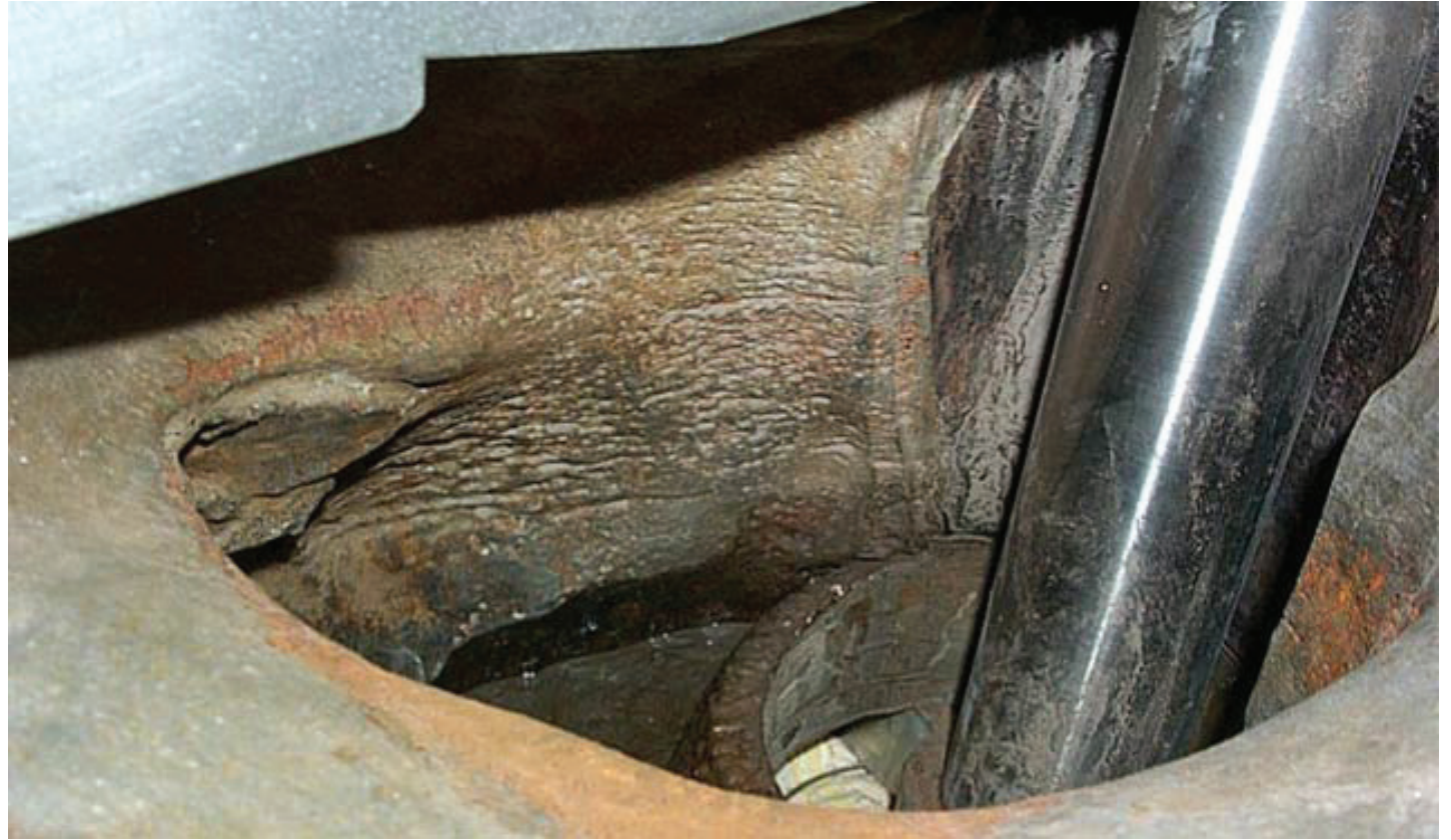
Result of boric acid corrosion. Image credit: https://www.nrc.gov/reactors/operating/ops-experience/vessel-head-degradation/vessel-head-degradation-files/looking-back-toward-nozzle3.html .
