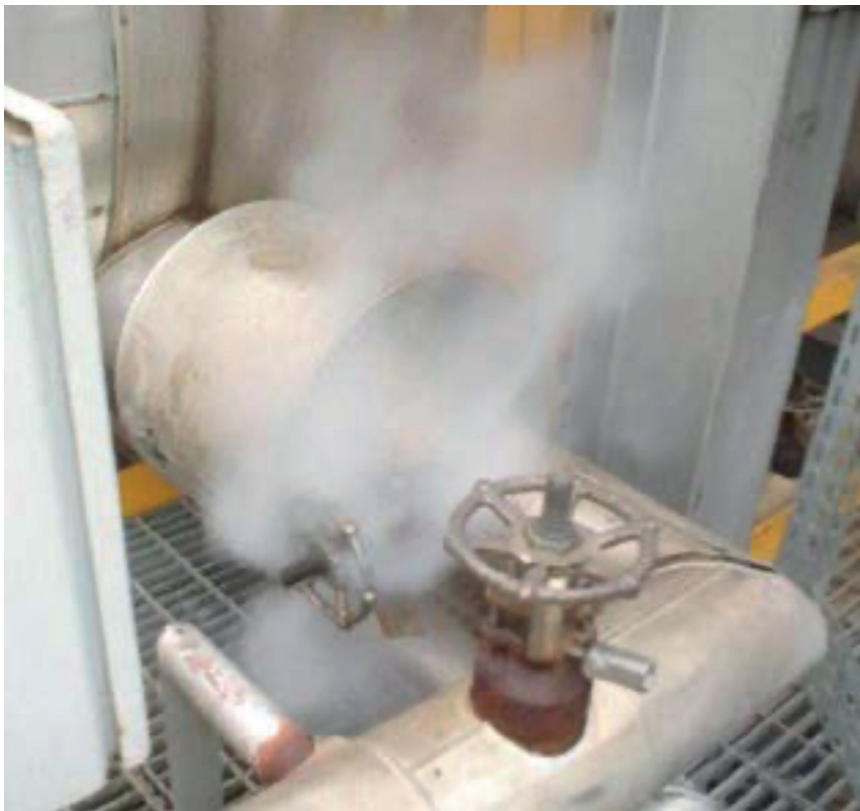
Before the use of reinforced packing.
